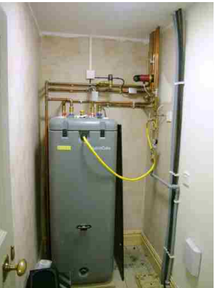
Hygienic hot water store
