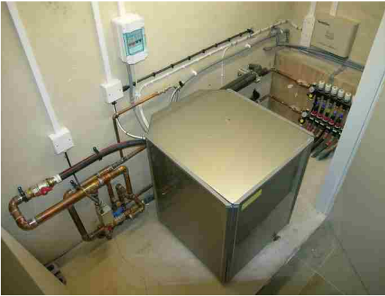
Heat pump & manifold 1 of 3
